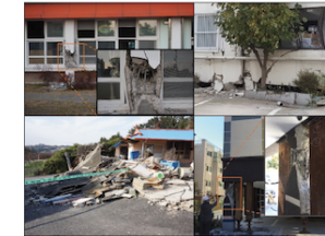
Structural Damage Due to the 2017 M5.4 Earthquake near Pohang City, Korea
